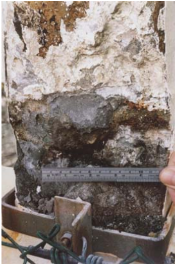
Figure 6: Breakout of Hanger N19 in 2002. Original flat bar reinforcement had disintegrated in to a fine black dust without expansive product.
