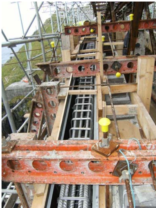
Figure 21: Southern rib arch reinforcement. The original rib is visible on the right hand side.
