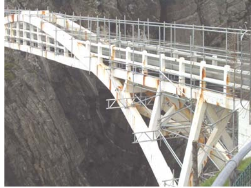
Figure 9: Temporary access scaffold supported directly from the arch ribs erected in June 2005.
