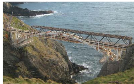
Figure 15: Erection of the temporary truss. All of the members were delivered and erected by hand.
