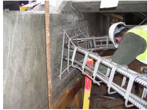
Figure 27: Fixing the reinforcement for the arch rib braces. The stainless steel couplers are visible.
