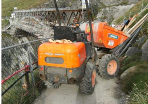
Figure 12: This four-wheeled articulated mini-dumper was the largest plant size which could access the site. There was no space to turn the machine and it was driven down and reversed up the steep access paths for the duration of the works.
