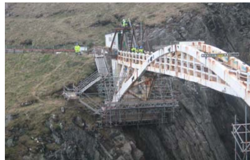
Figure 14: The existing arch ribs supporting the access scaffold in the back spans and supports to the existing deck.
