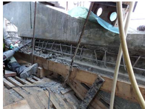
Figure 28: Preparing the joint between the deck and the arch at the quarter span.
