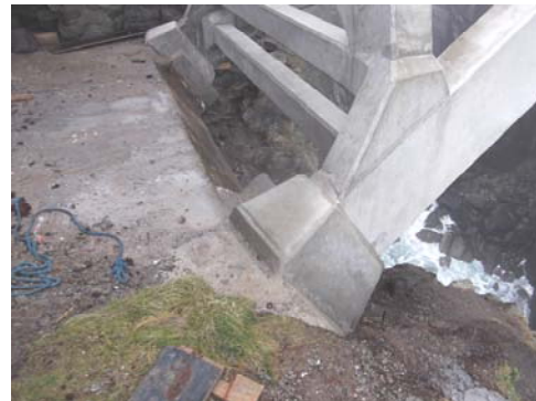
Figure 29: Completed bearing detail with the original arch rib springing points remaining in place.
