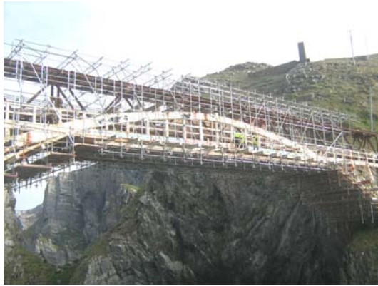
Figure 16: The access scaffold supported from the temporary truss and the temporary deck supported from the existing arch ribs.
